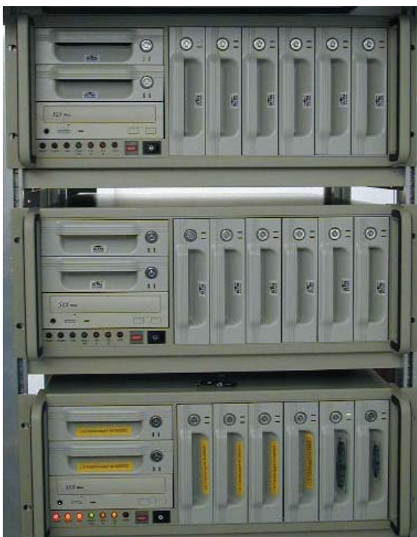
Figure 2: This figure shows three of the NGAS units mounted in a rack. They are fully equipped with eight disks each, giving a total of 1.65 terabyte of on-line storage capacity with three processors running at 1.2 GHz each.
