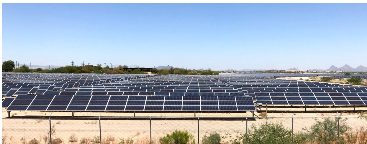
Figure 2.4: Single-axis tracking solar panels at the University of Arizona Tech Park in Tucson, Arizona.
